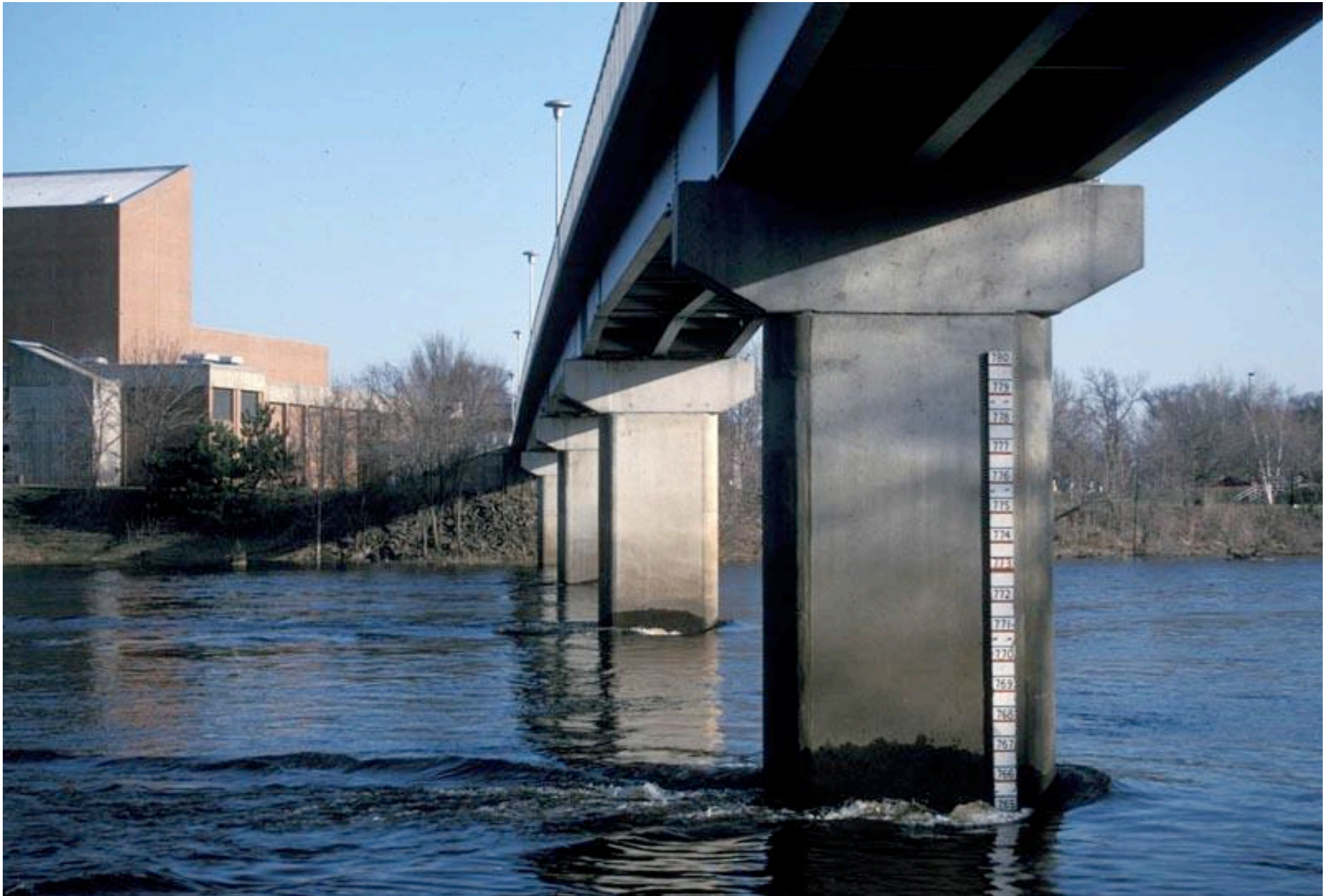
Stream gauge on bridge support, Chippewa River, Wisconsin
