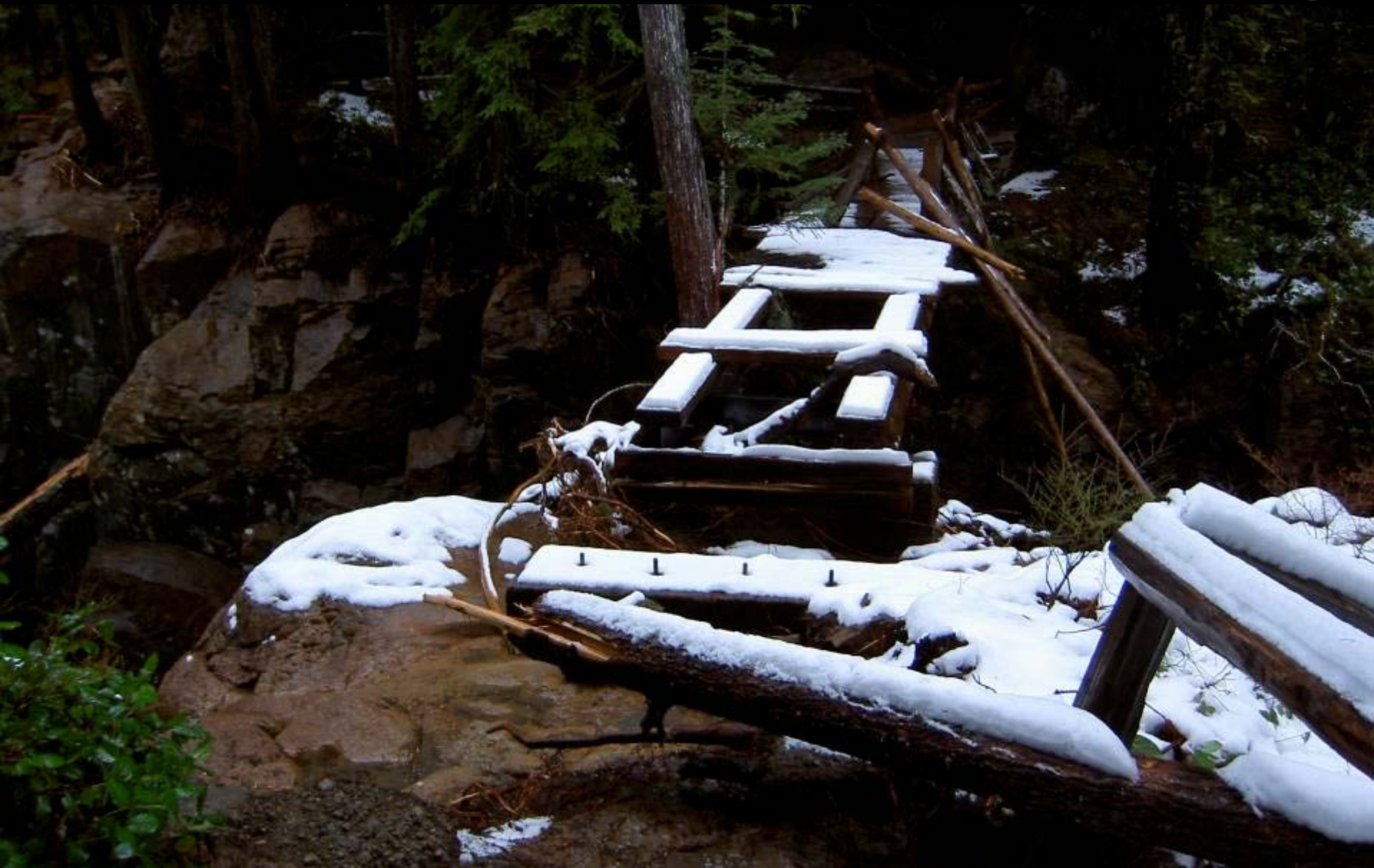
The Silver Falls bridge was heavily damaged
