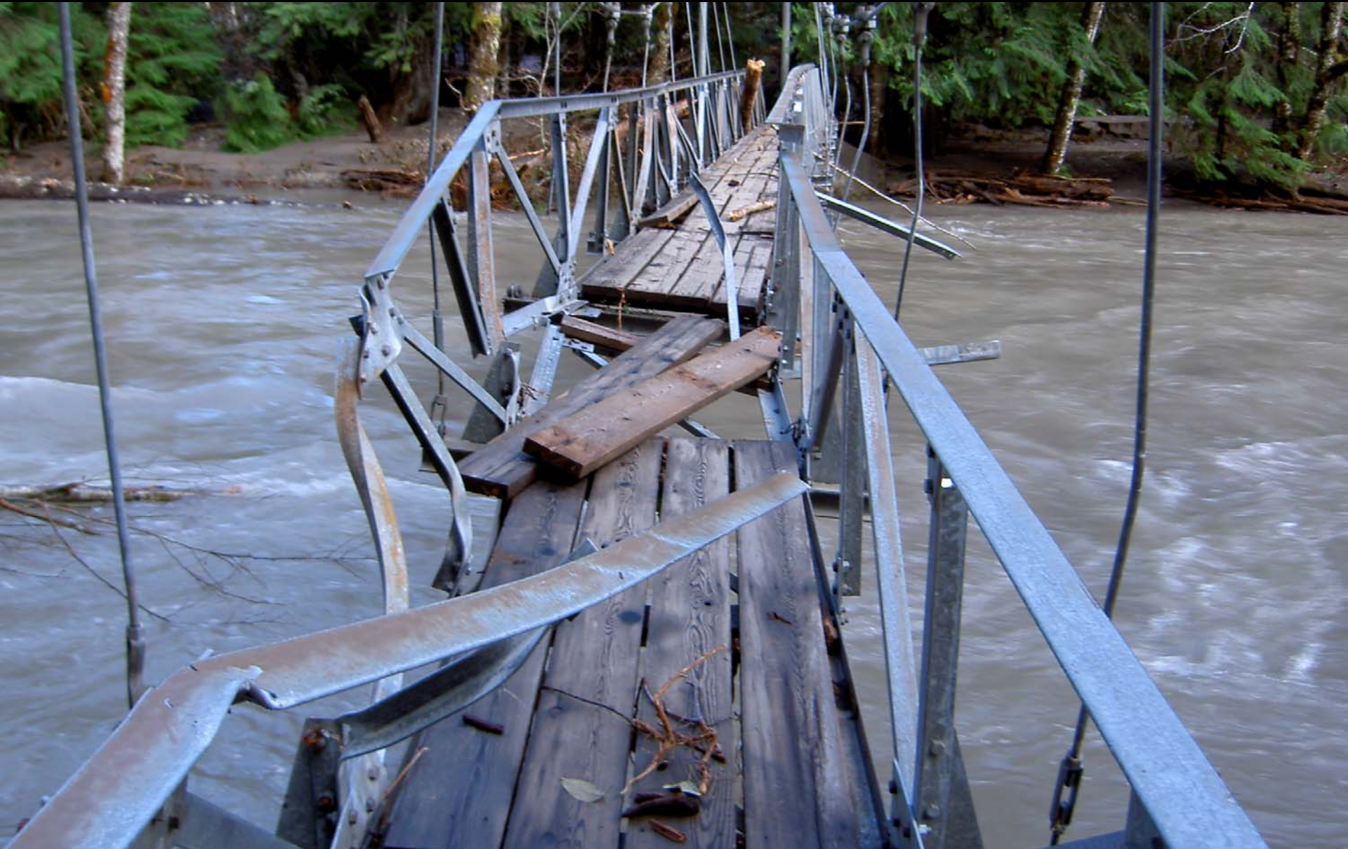
The damaged suspension bridge
