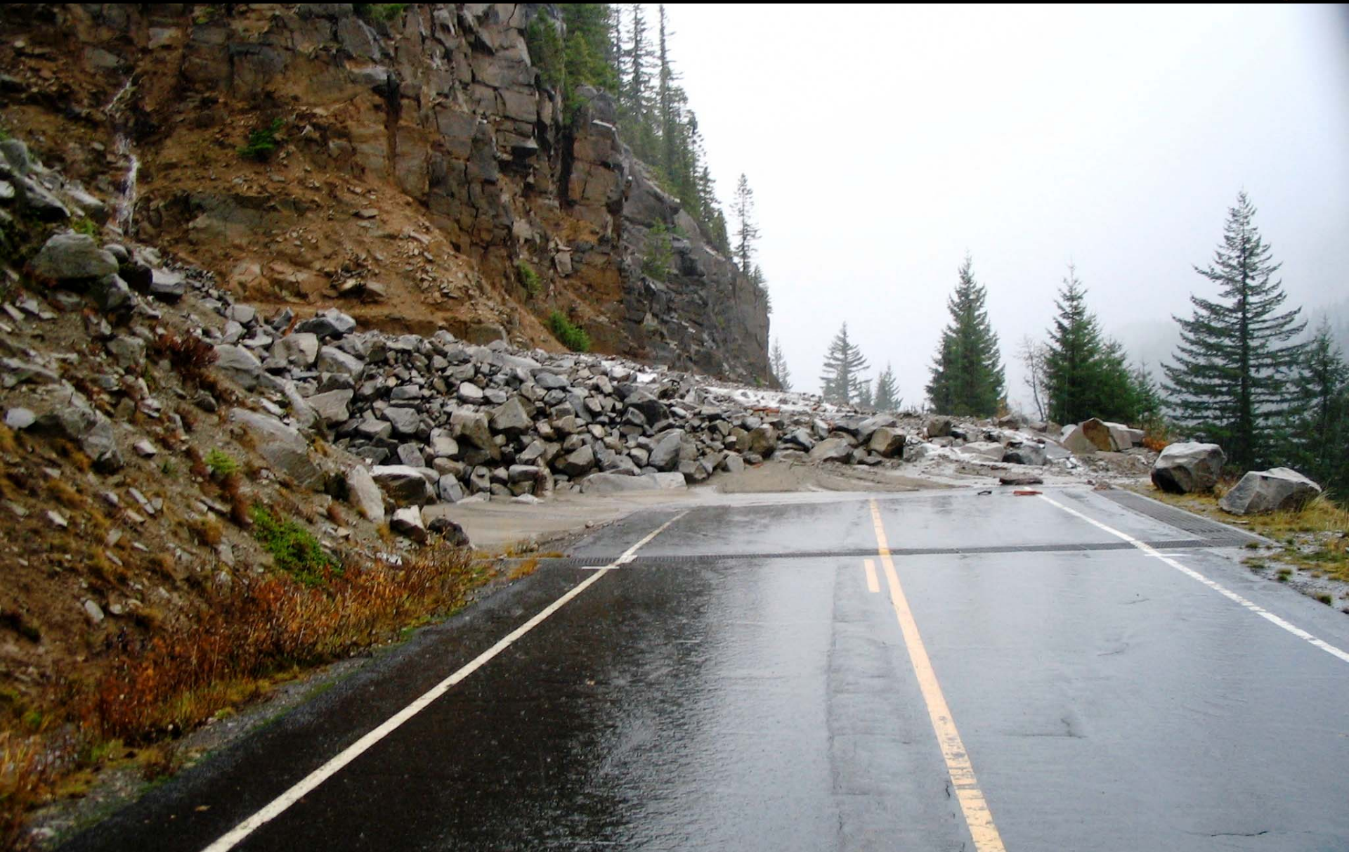
Landslide above Glacier Bridge on the Paradise Road
