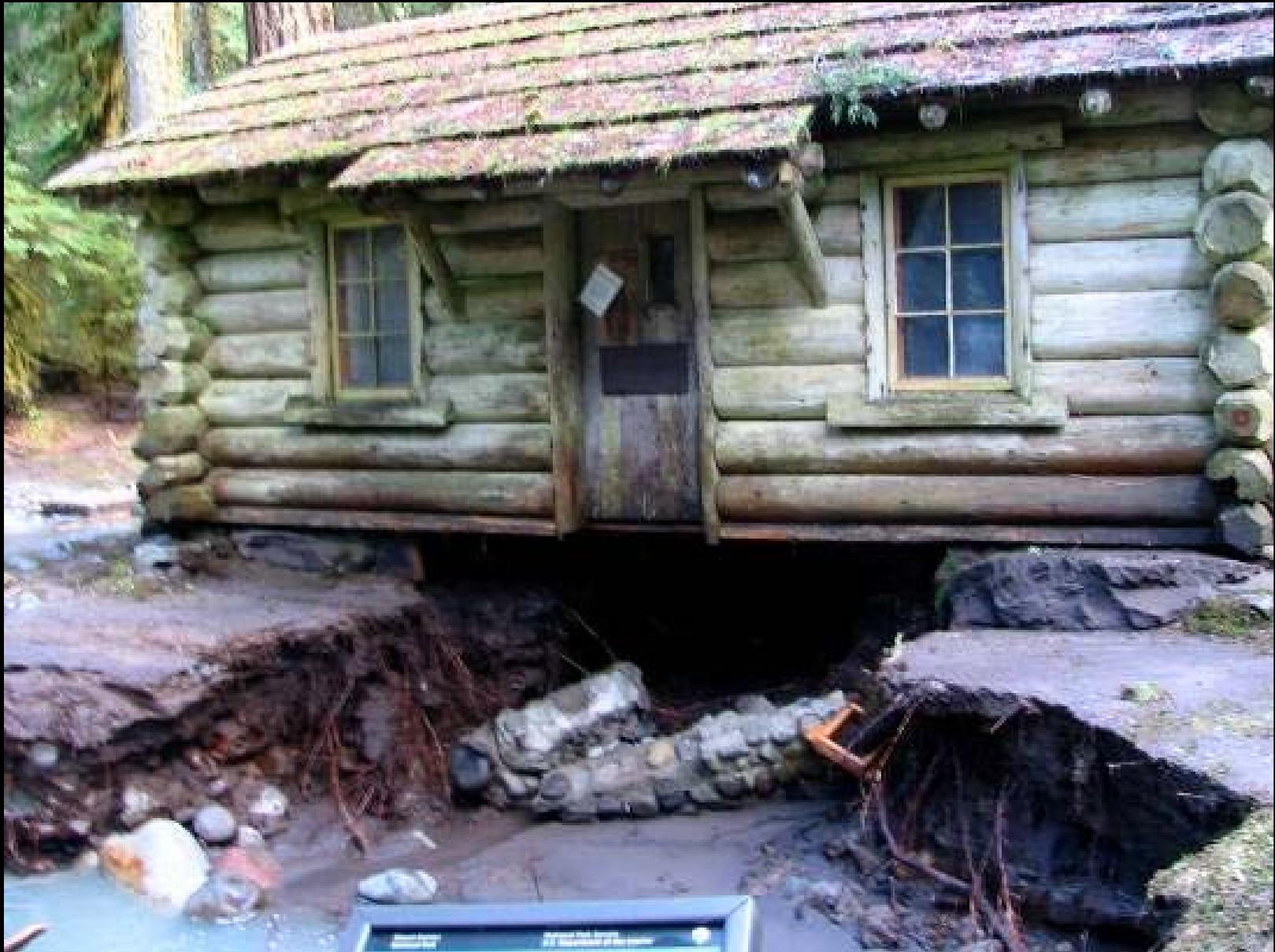
The historic Ipsut Creek Cabin was undercut by the river
