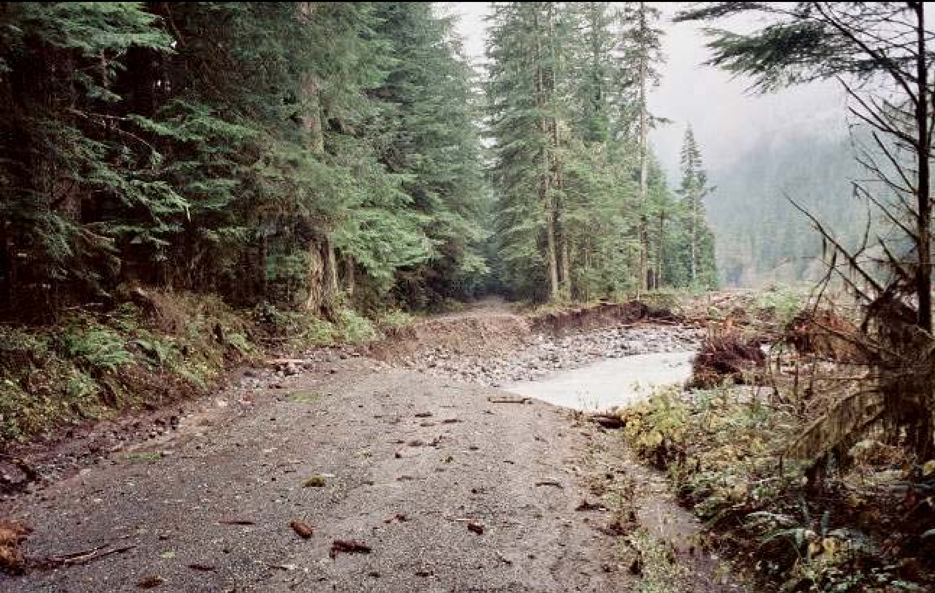
One of several gaps in the road near Ipsut Creek
