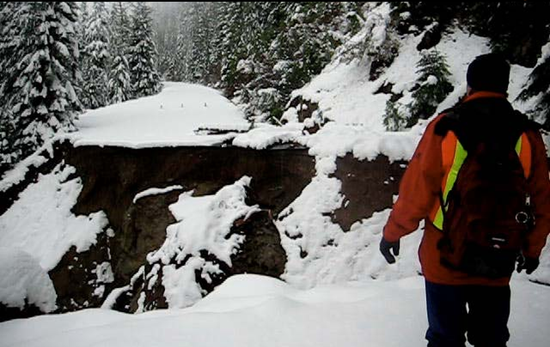
Inspecting the damaged road
