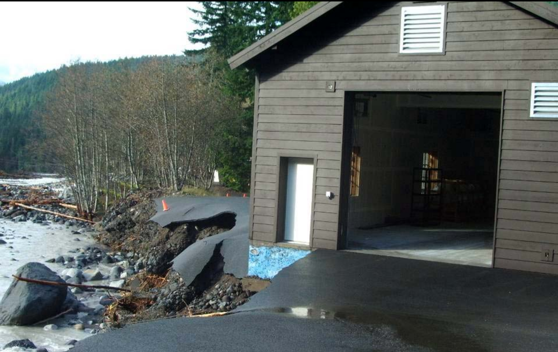
The Emergency Operations Center after the flood. The parking lot is destroyed.
