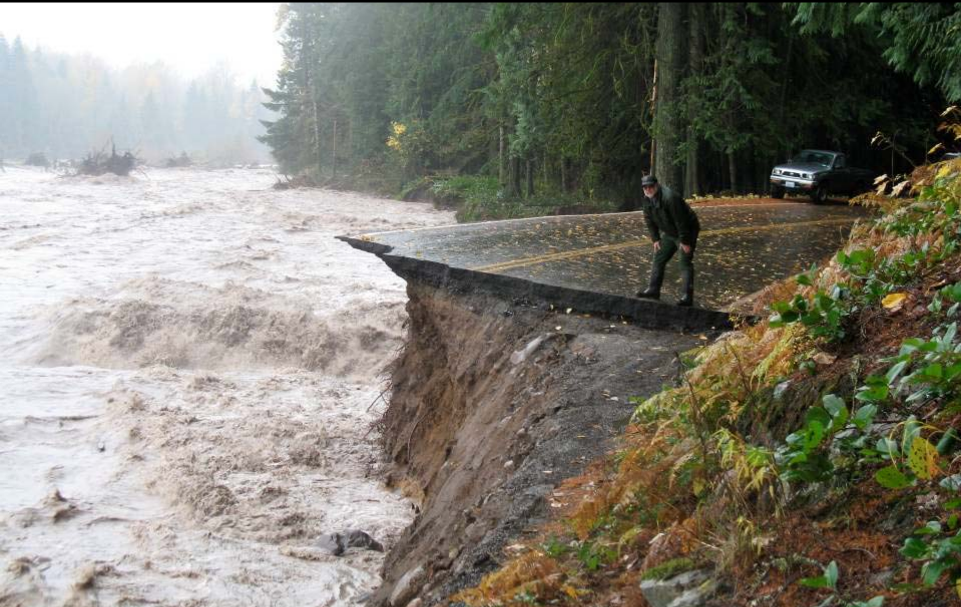
The broken edge of the Nisqually Road
