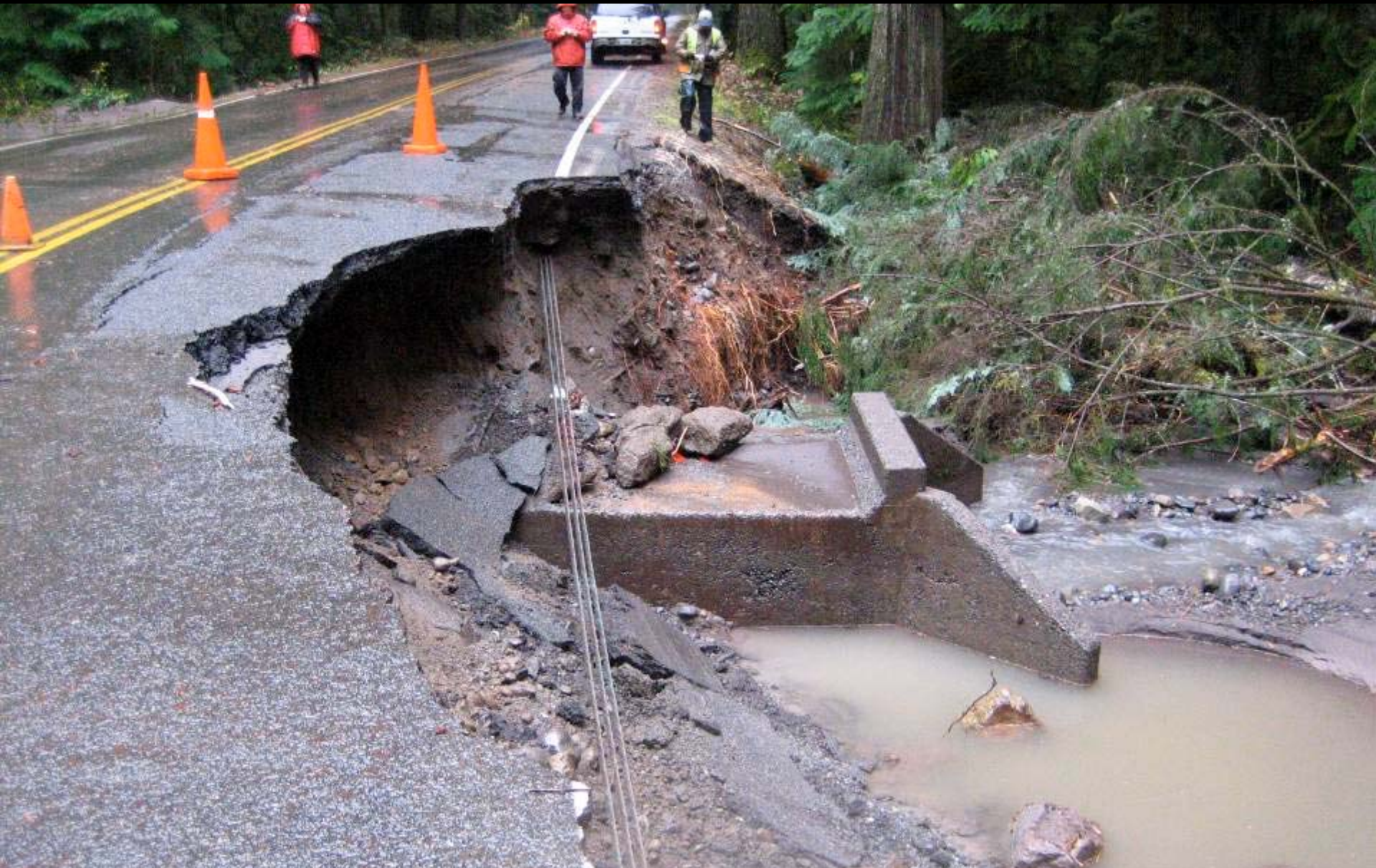
Damage to the Nisqually Road across from the Westside Road junction
