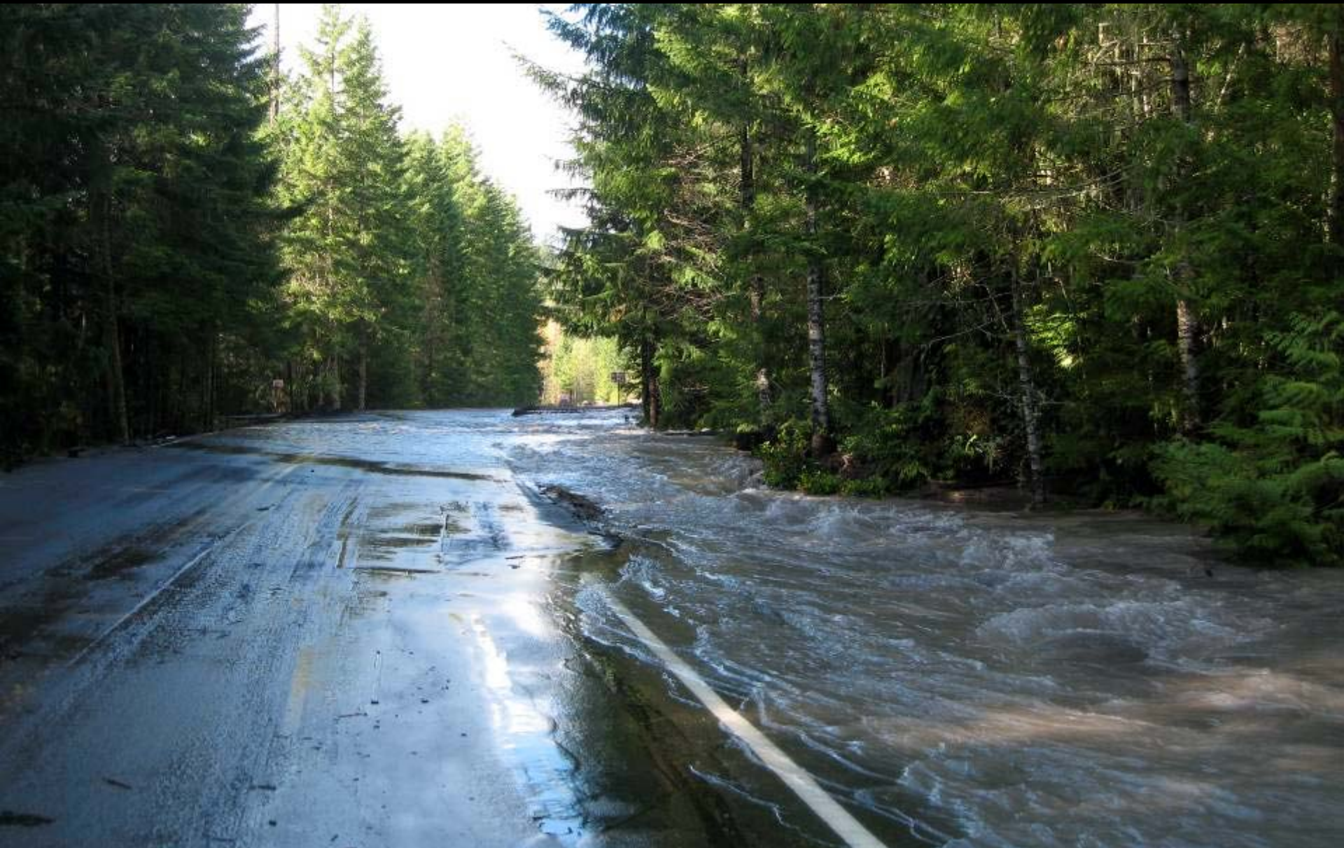
Kautz Creek continues to erode the edges of the Nisqually Road
